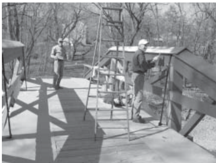
The Friends’ volunteer painting crew, (from back to front) Bill Trainer, Tom Williams, Gordon Heisler and Pete Sperry ( not shown because he was busy taking the picture) worked diligently on the Thompson Neely Bridge. And no, Tom Williams, shown lying on the bridge deck, wasn’t sleeping on the job – just trying to get to a hard to reach spot.
